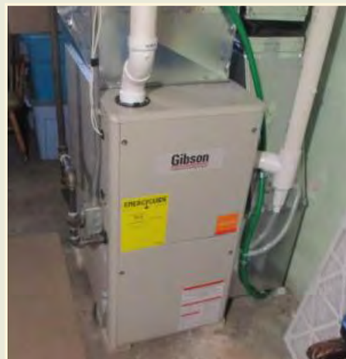
A newly installed furnace that will provide dependable heat for a household that experienced an emergency situation last winter.
