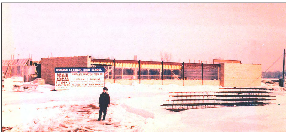
Construction of Oshkosh Lourdes High School is shown in progress in February 1959.
