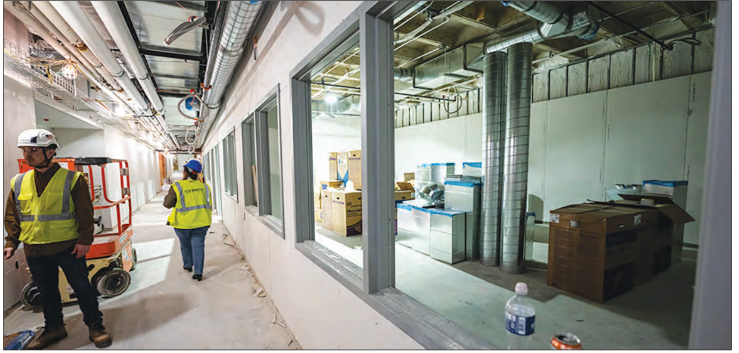
Construction work continues in Clow Hall. The project is now expected to wrap up in July. The upgrades to Clow Hall, which began in spring 2022, are more than a decade in the making.
