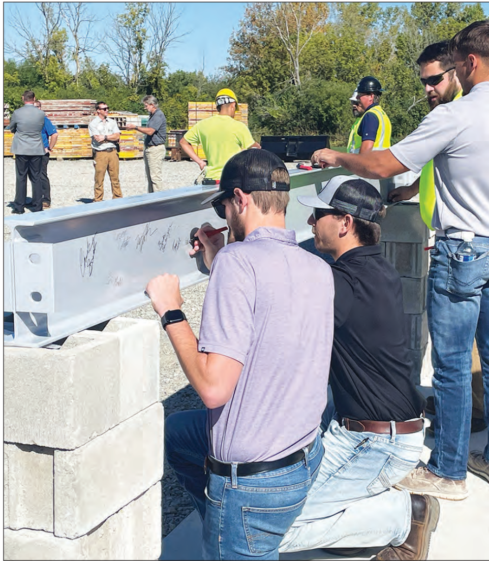
FVTC staff, students and supporters were invited to sign the final steel beam before it was lifted into position at the new construction training site on Waupun Road.
